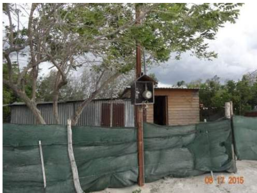
Image 14: Open meter box and exposed wires.
